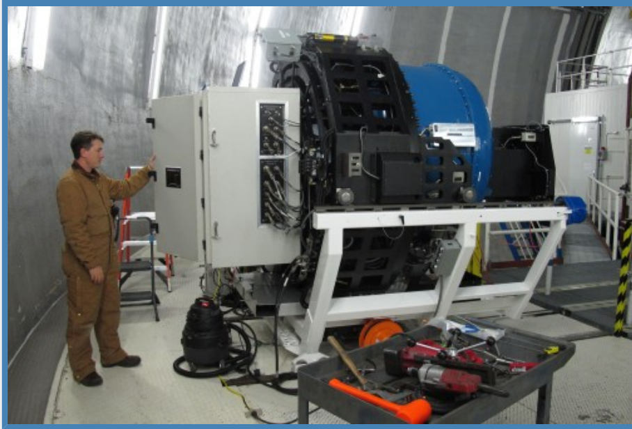
Figure 1. WMKO Support Astronomer Marc Kassis inspects the electronics cabinet at the rear of MOSFIRE shortly after its delivery to the Keck I telescope's Nasmyth deck.
