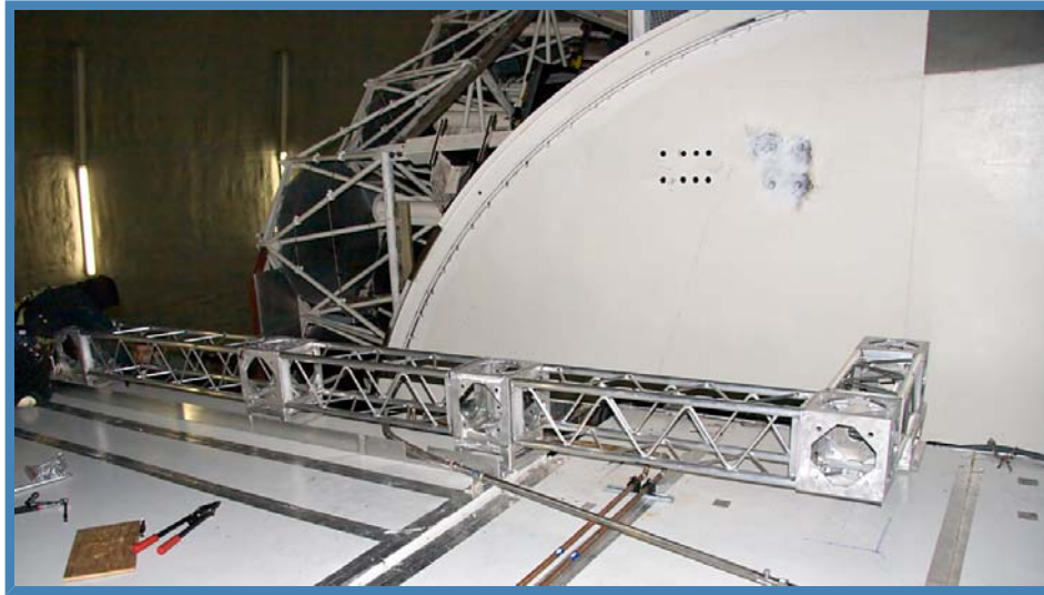
Figure 2. Free-space transport (FST) truss structure being installed on top the laser and HIRES enclosures. The truss will support some of the FST relay mirrors and beam containment tubing. The Keck I elevation ring is in the background.
